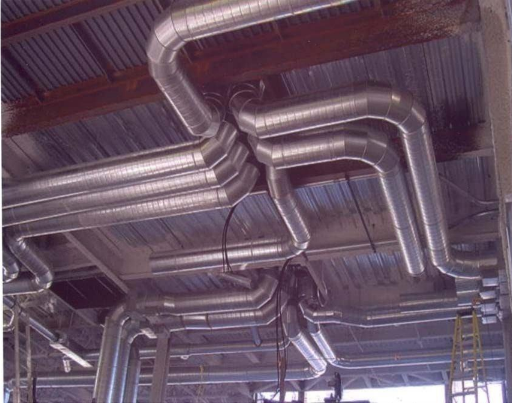
Fig 5 Duct design Photograph
